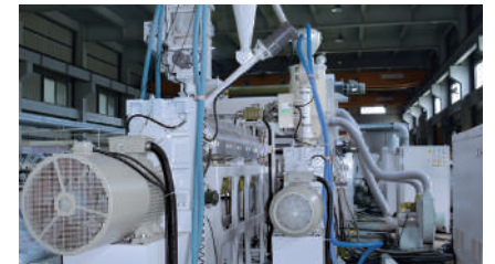
The double extrusion goes through the feed block device and the special T-die runner to make the three-layer A.B.A co-extrusion.
